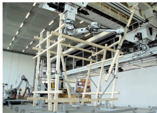
The CantiBox under construction at the Robotic Fabrication Lab at ETH Zurich in 2022.
